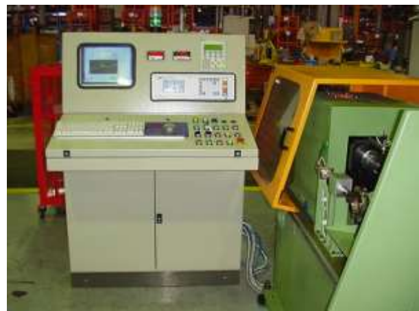
- Example of installed quality control system (gearboxes) -
